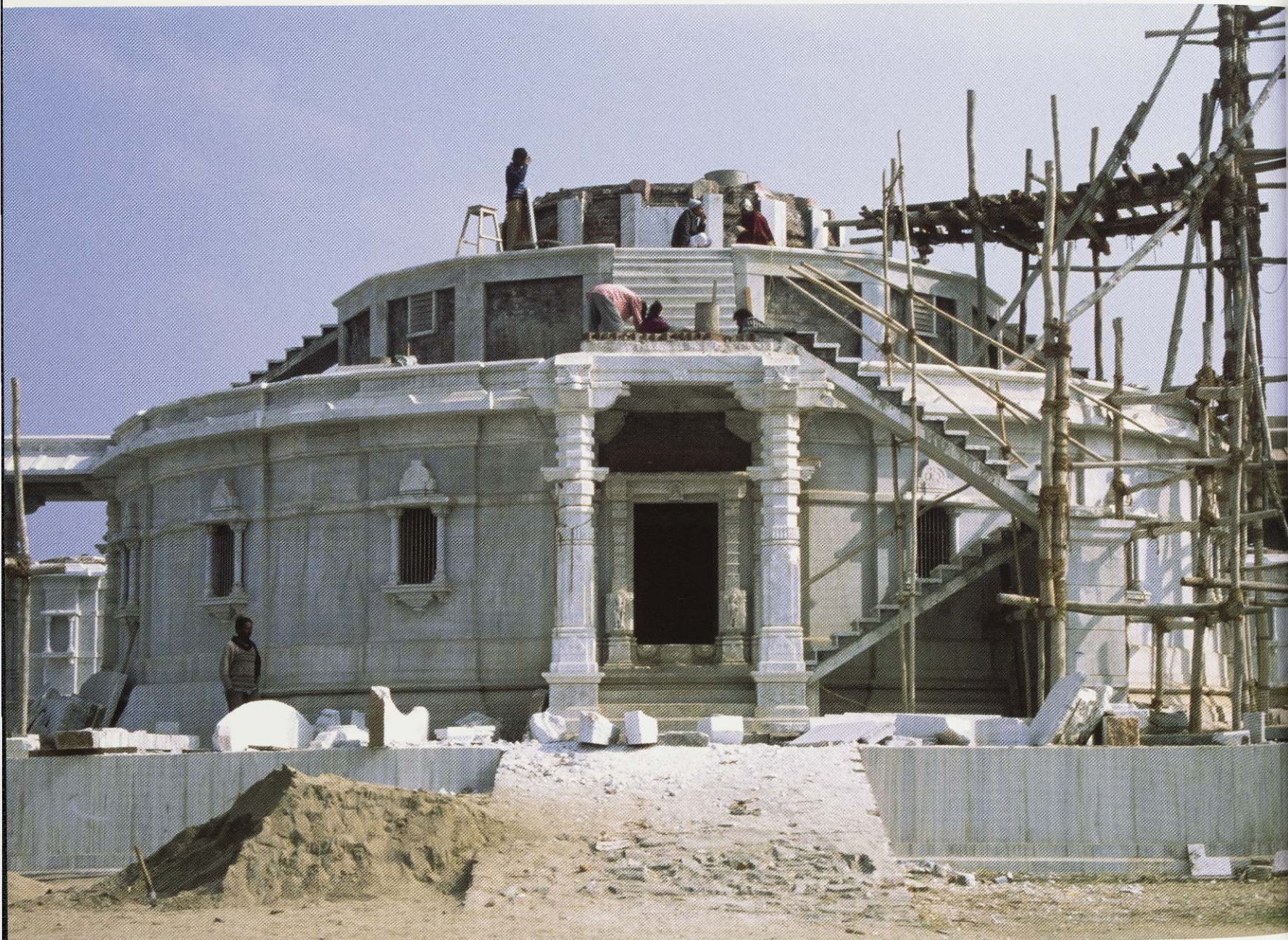
572. The Śrī Samavasaraṇa Mahā-mandir Tīrtha, a large-scale mythical teaching auditorium of the Jinas, under construction at Himacal Surya Nagar in 1998.
