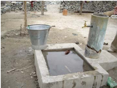
Figure 6.4 Water tap from WASEP in Bukyalpa with broken concrete casing
