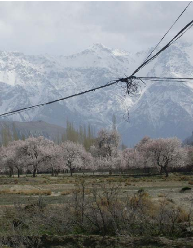
Figure 3.3 Provisional connected power cables Photo: Altenkirch 2008
