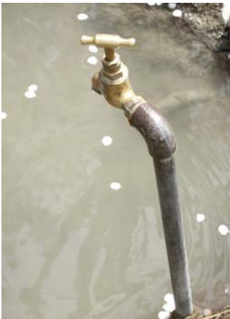
Figure 6.3 Water tap from WPD in Bloqkhor
