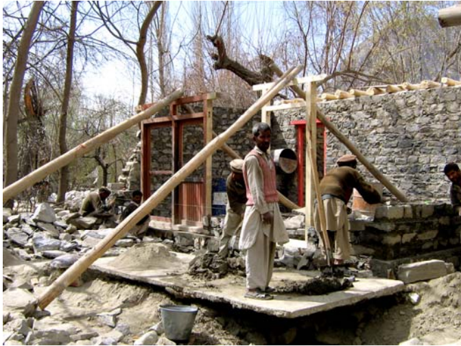
Figure 8.5 Construction site of a new hotel in the central section of the bazaar area Photo: Piel 2008
