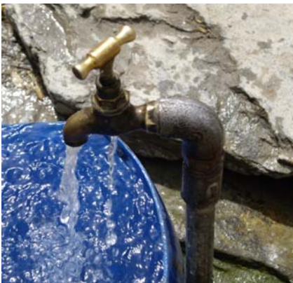
Figure 6.7 Complete and working tap in Gongma Xserdrong
