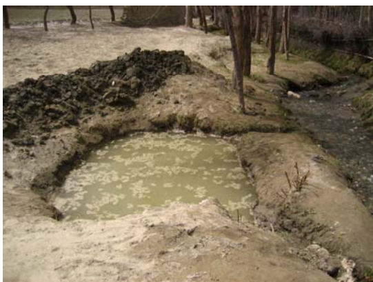
Figure 5.4 Sediment trap filled with water. Photo: Dieckhoff 2008
