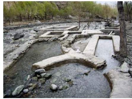
Figure 6.2 Intake point at the nālā for the water supply system in Shigar
