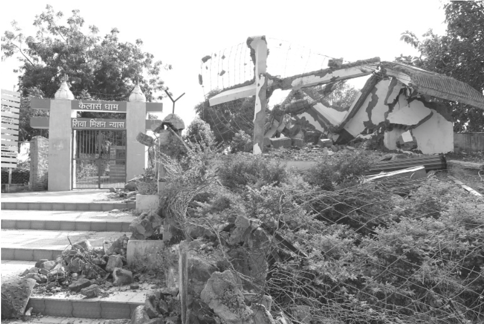
Plate 44.2: Entrance to the Śiva Miśan Nyās with the demolished “Mantra Bank” building.
