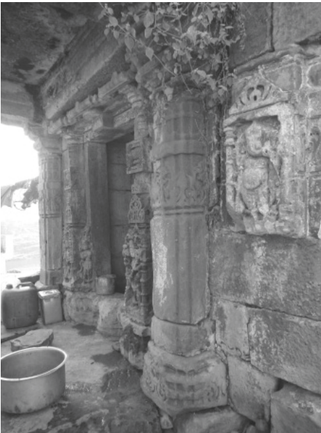
Plate 76.2: Shrine No. 2, front wall with entrance to garbhagrha and sculpture of Gaṇeśa.
