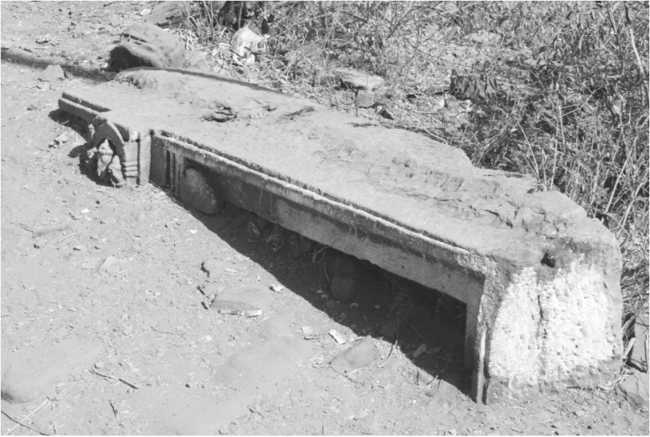
Plate 21.4: Loose door lintel, south of the Bhīmārjunī gate.
