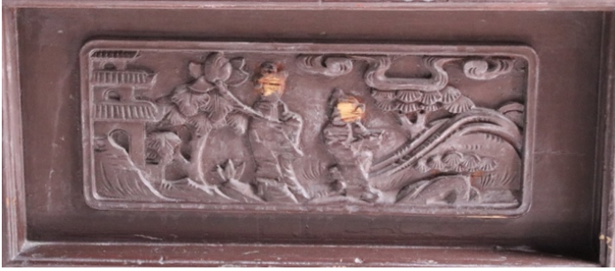
Figure 4-25. Scratched Wooden Carving on Partition Wall.
