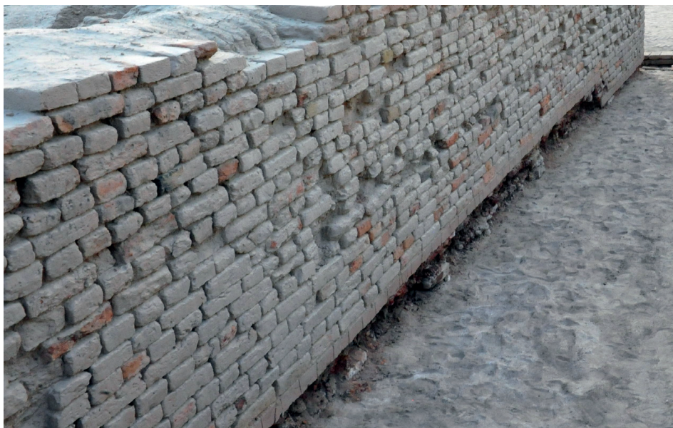
Fig. 10. Salt damage in Mohenjo-dāro
