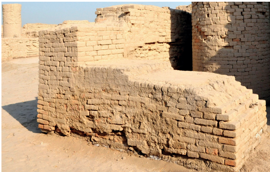
Fig. 9. The impact of saline soil on walls in Mohenjo-dāro
